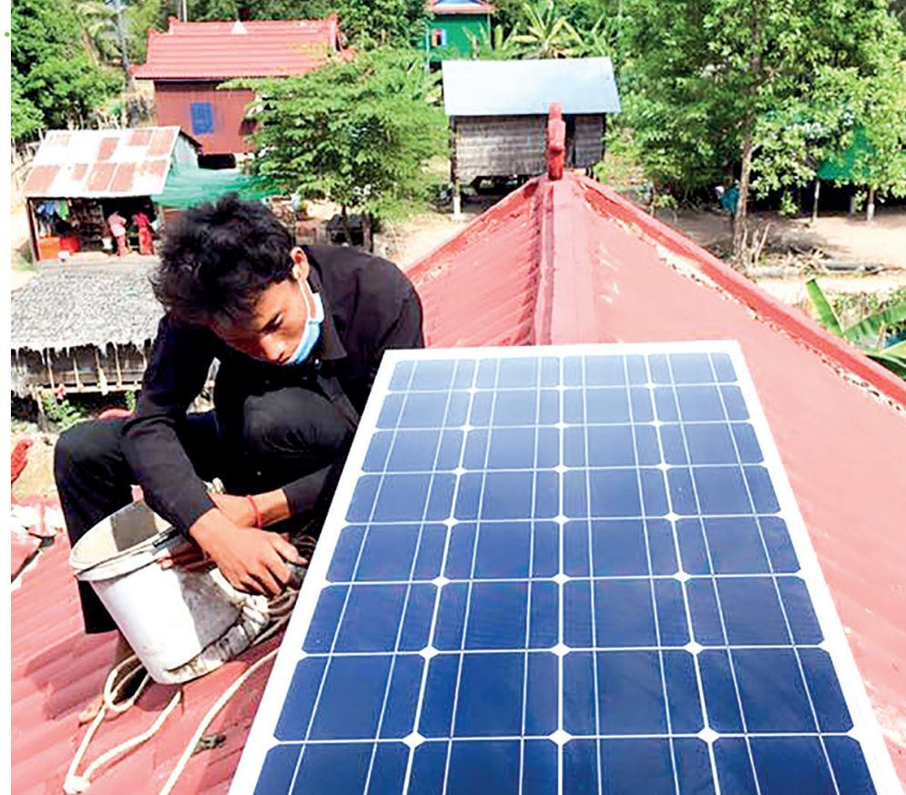
A solar panel being fixed by NRG Solutions solar company on the roof of Suon Dyna's house.
