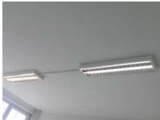
Figure 6: New surface mounted luminaries
