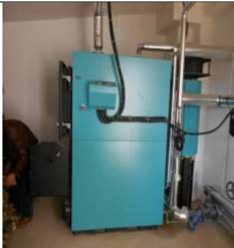
Figure 3: Energy efficient boilers
