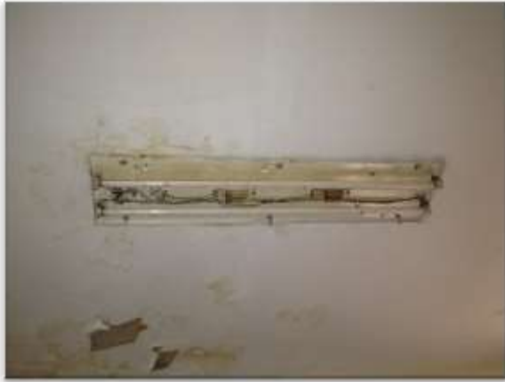
Figure 5: Surface mounted luminaries AFTER EEM EE MEASURES
