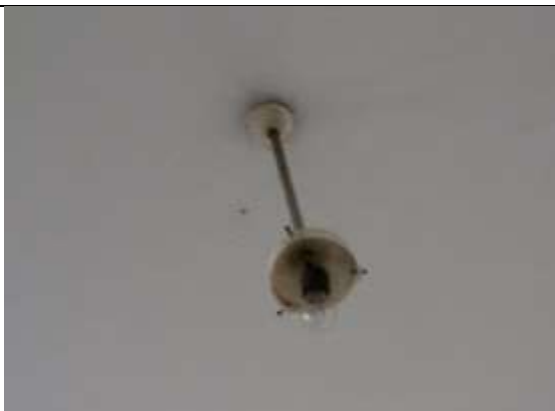
Figure 5: surface mounted luminaries
