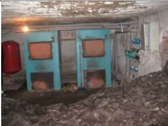
Figure 3: Wood and coal Boilers
