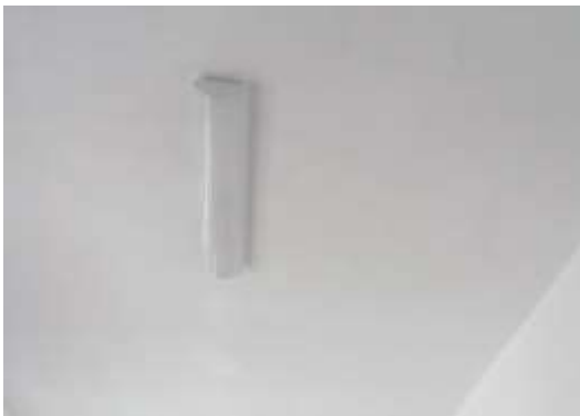
Figure 5: New surface mounted luminaries
