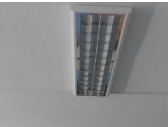
Figure 5: New surface mounted luminaries
