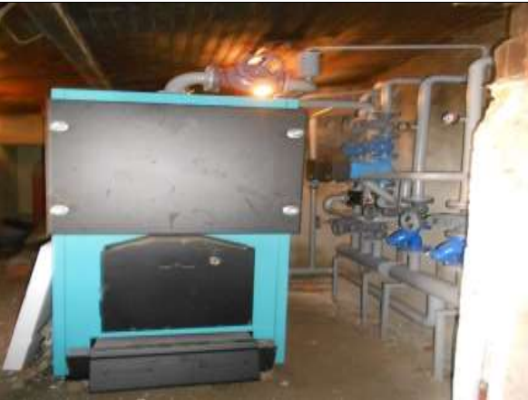
Figure 3: Energy efficient boiler
