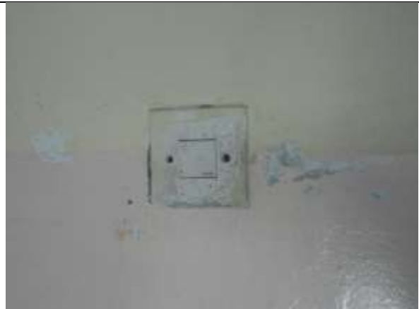
Figure 6: old electrical switch
