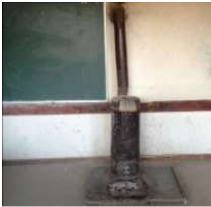
Figure 3: Existing stoves Electrical installation
