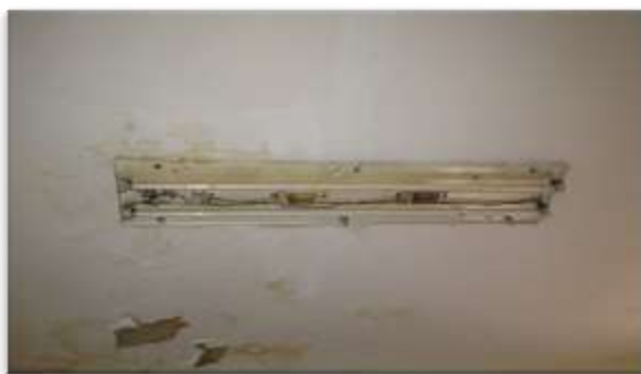
Figure 5: Surface mounted luminaries
