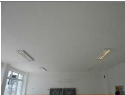
Figure 5: New surface mounted luminaries
