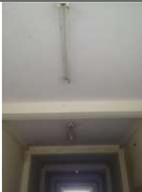
Figure 5: Surface mounted luminaries
