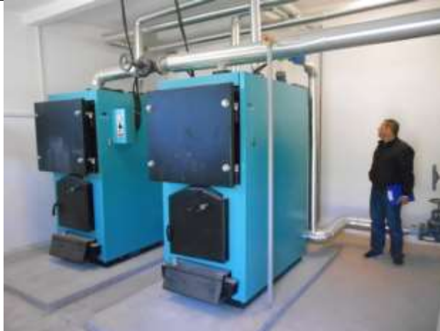
Figure 3: Energy efficient boilers
