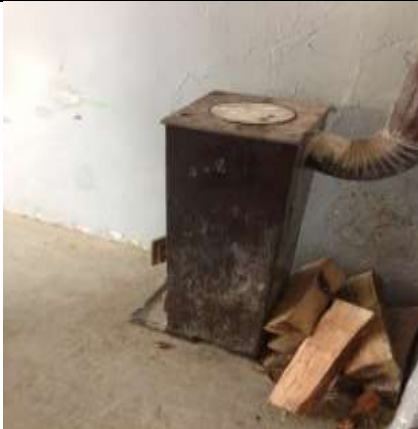
Figure 3: Existing wood stoves
