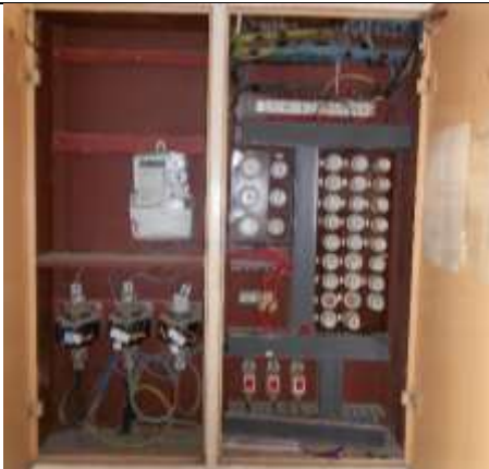
Figure 5: Existing Distribution Board
