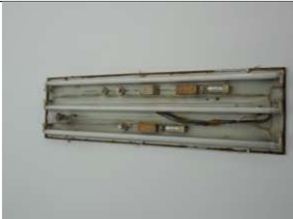
Figure 5. surface mounted luminaries
