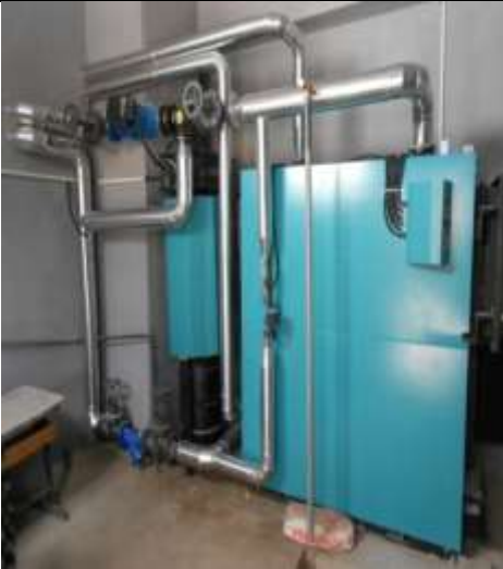
Figure 3: Energy efficient boilers
