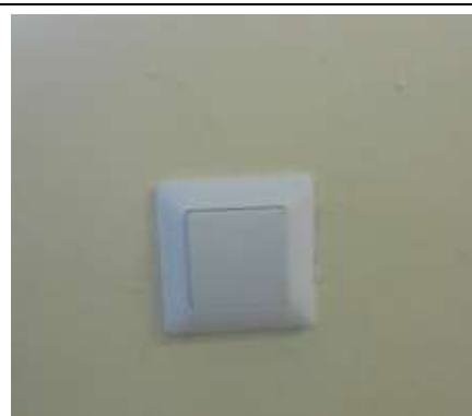
Figure 6: New manual switch
