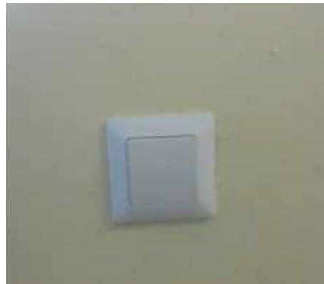
Figure 6: New manual switch
