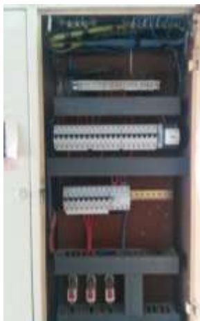
Figure 5: New manual switches
