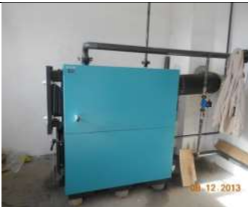
Figure 3: Energy efficient boilers
