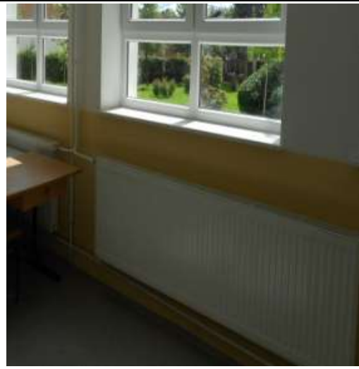
Figure 4: New radiator , refurbished installation
