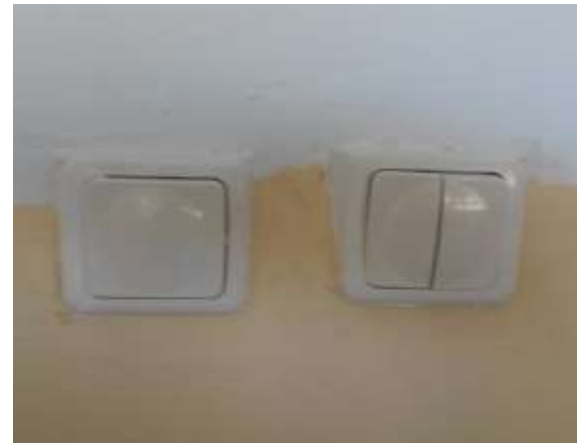
Figure 6: new electrical switches
