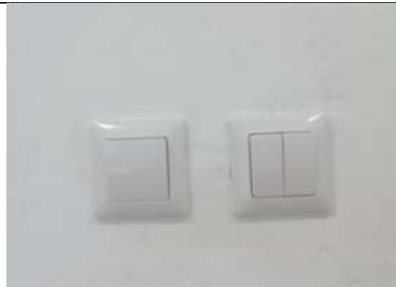
Figure 6: New manual switch
