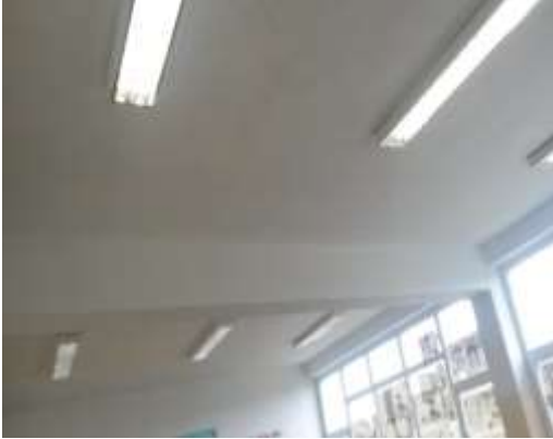
Figure 5: New surface mounted luminaries
