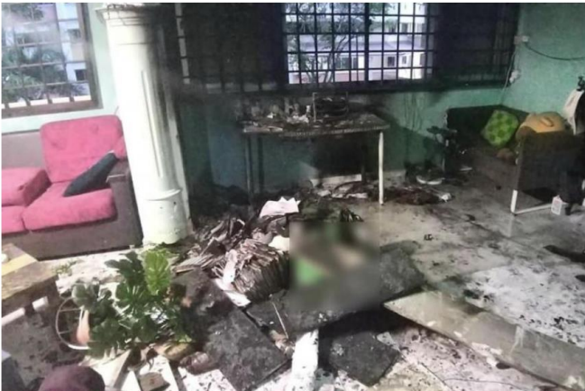
The fire involved a battery pack of a power-assisted bicycle at Block 723 Jurong West Avenue 5. PHOTO: SINGAPORE CIVIL DEFENCE FORCE/FACEBOOK
