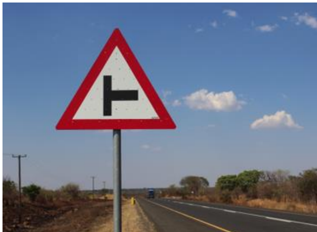
Perforated signs as a measure to protect against vandalism – only partially successful
